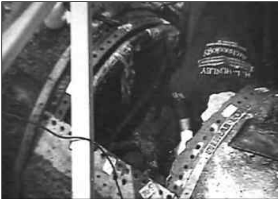
To reach the inside of the submarine, some cover plates were removed. The rivet holes are clearly visible.
